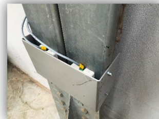
Figure 8 – Strain gauge (with anti-shock protection) installed in the base of the column.
