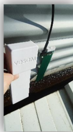
Figure 5 – Gutter sensor in the roof of the industrial unit.
