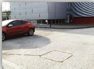
Figure 7 – Inductive loop for traffic control.
