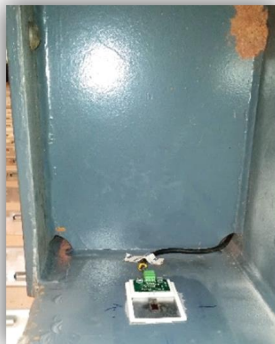
Figure 6 – Installation of strain sensor on the bottom flange of the main girder.
