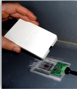
Figure 6 – Installation of strain sensor on the bottom flange of the main girder at mid-span.
