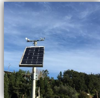
Figure 9 – Weather station with energy harvesting system (solar power).
