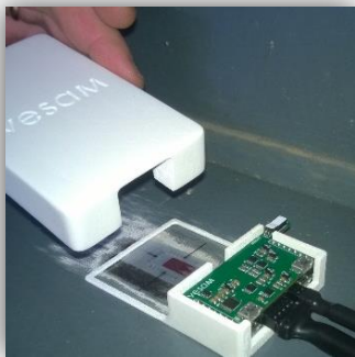
Figure 7 – Installation of OneSensor (strain gauge, accelerometer, temperature and relative humidity sensors all-in-one).
